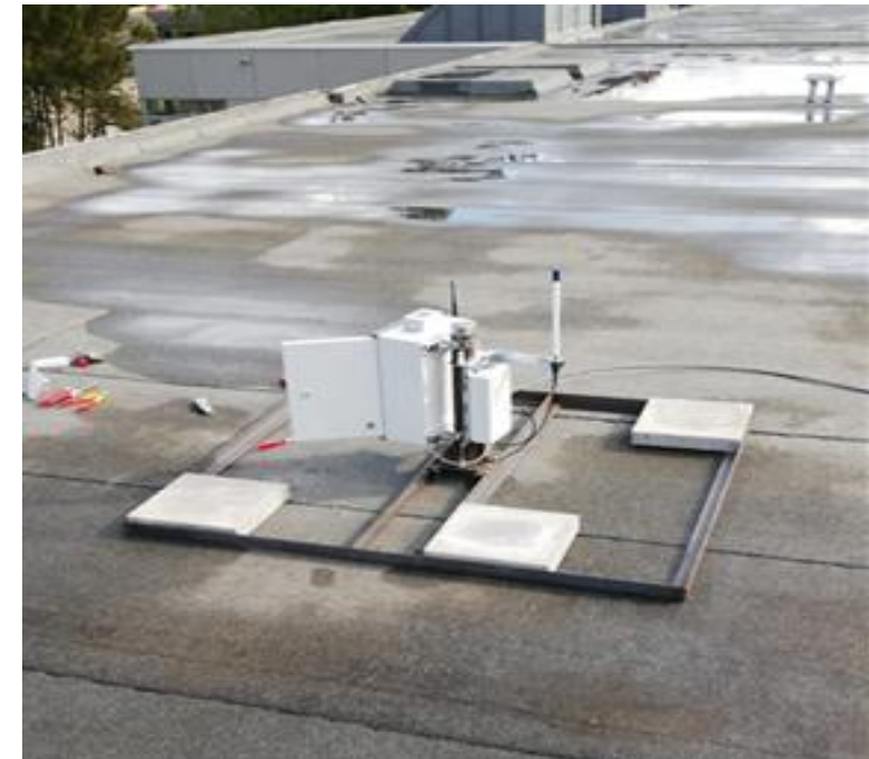
Gateway (installed on a school roof)
